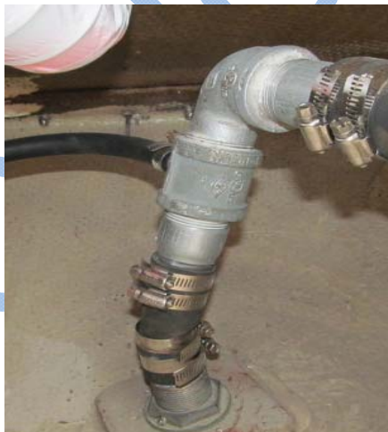
Buckled exhaust hose at throughhull
