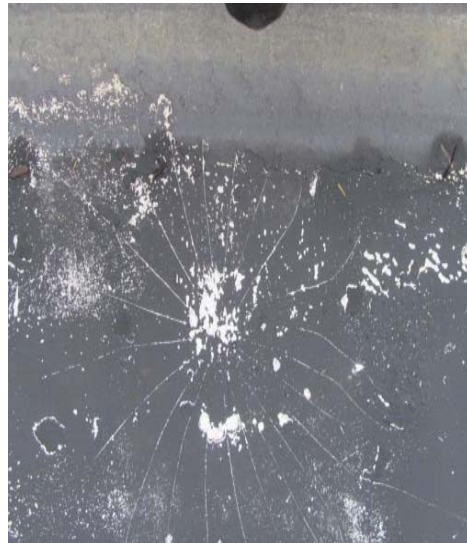
18" star fracture on transom
