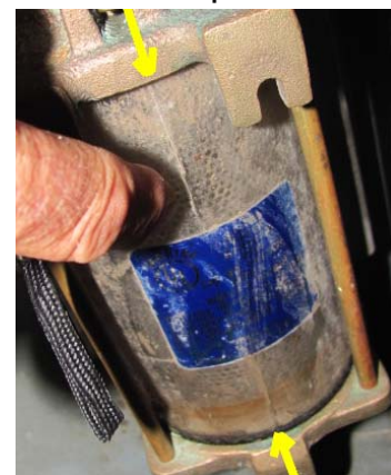
Cracked strainer cylinder
